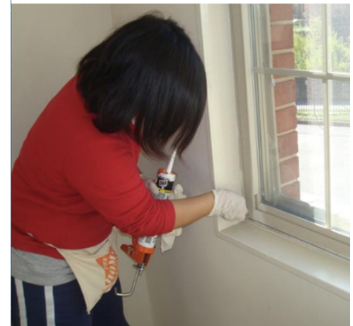
Patch cracks around windows.
