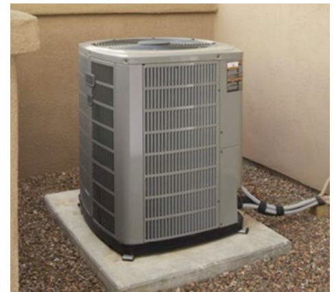
Upgrade HVAC systems with efficient models that do not use CFCs or HFC refrigerants
