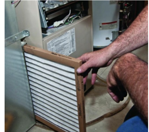
Dirty air filters can seriously cut HVAC efficiency
